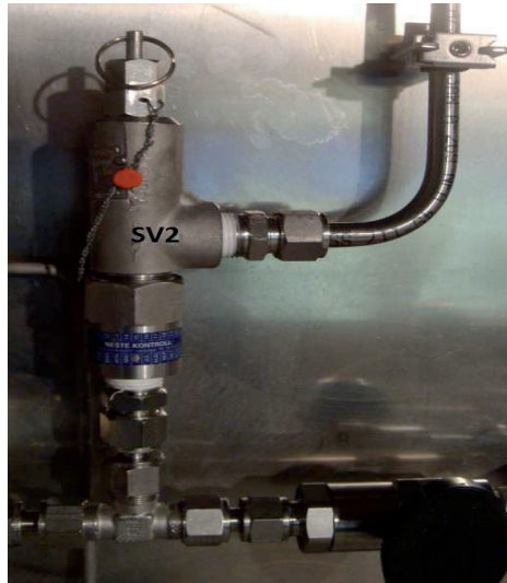
Figure 2- 8: Safety Relief Valve SV2 (close-up view)
