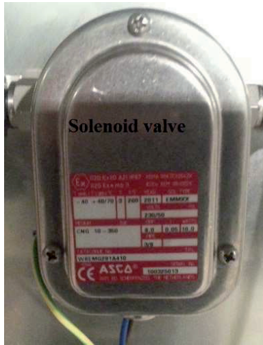
Figure 2-9: Solenoid valve (close-up view)
