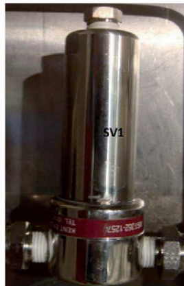
Figure 2-7: Safety Relief Valve SV1 (close-up view)
