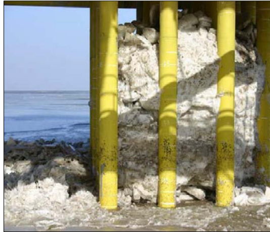
Figure 21. Sea ice pile-up between the platform legs in the Bohai Sea (Zhang and Yue, 2011)
