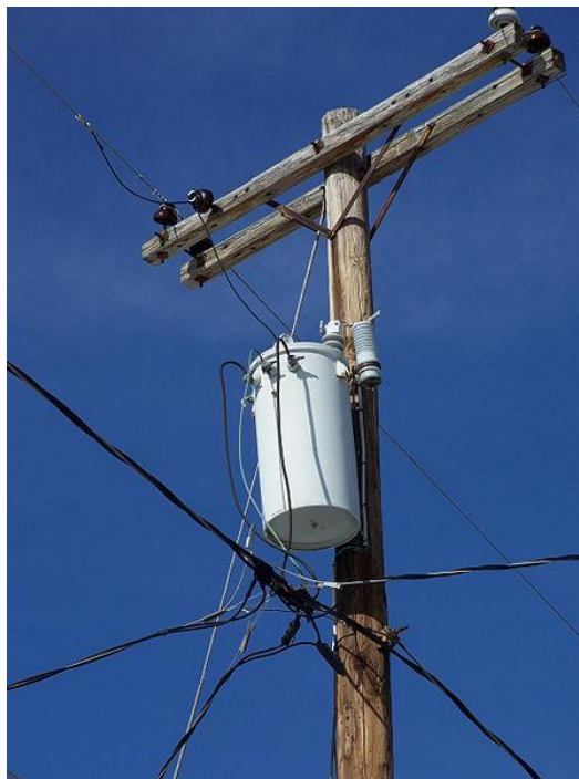
Figure 3 - Step-down transformer hanging on pole
