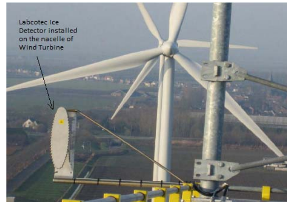
(a) Labcotec Ice Detector installed on the nacelle of wind turbine.
