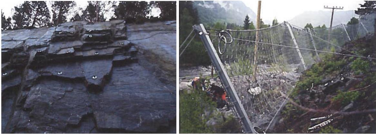
Figure 7: Bolting, a active rockfall mitigation measure (left). Rockfall catching fence, a passive rockfall mitigation measure (right). From (Domaas and Grimstad, 2014).
