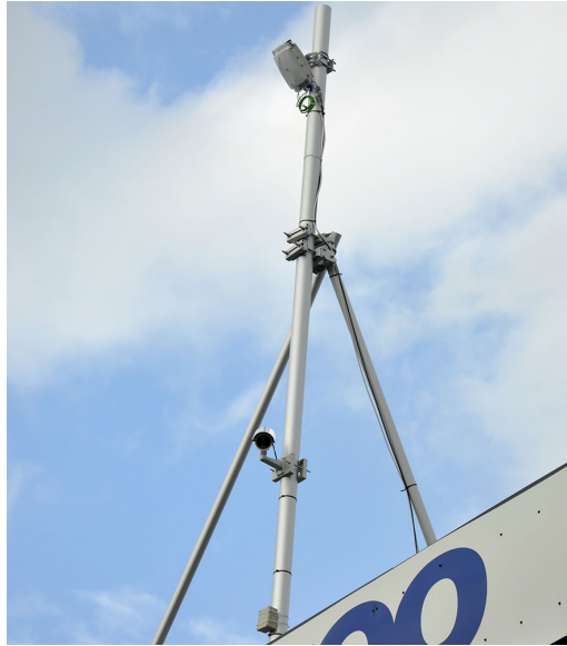
Figure 2.1: ZXY radio receiver mounted on antennas around Alfheim stadium
