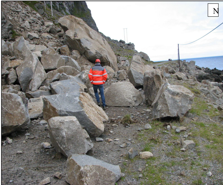
Fig. 19 Debris on the road, after the rock avalanche in 2011. The large boulder in front of the man is still in place, keeping the talus slope stable. Picture by Persson, SVV, 2011
