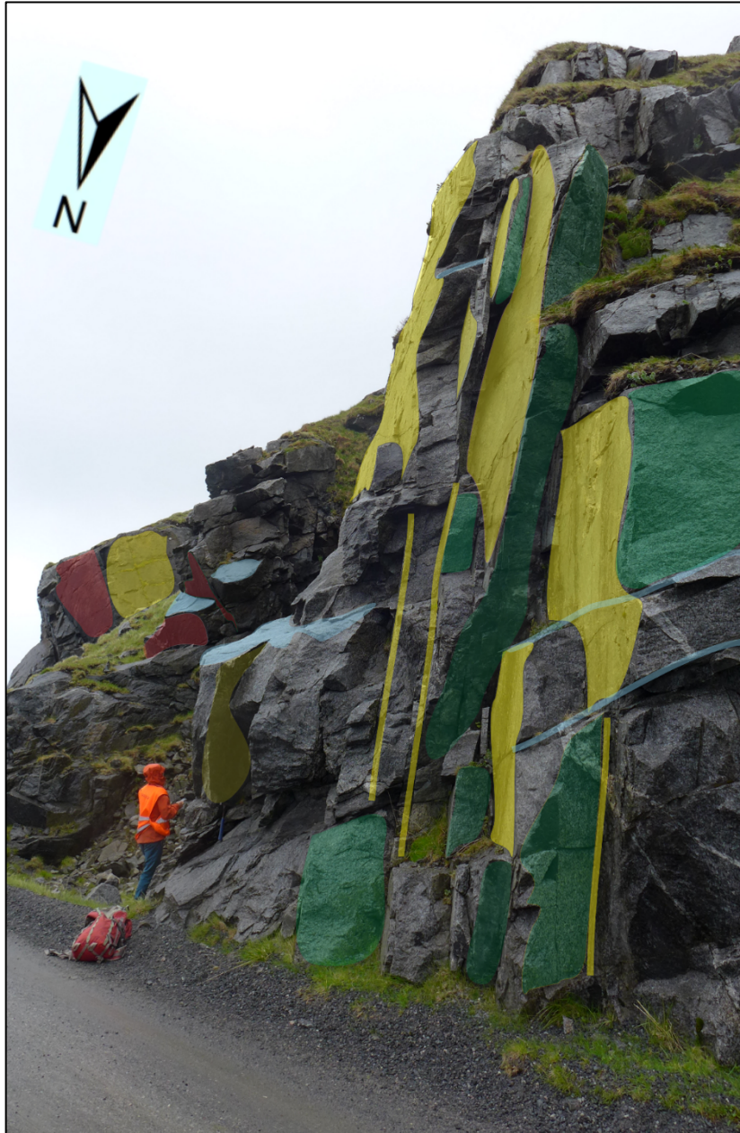
Fig. 46 Location 3, north of the UAV flight inspection area. The bedrock is weakly foliated and rather dominated by brittle fractures/joints. Surfaces are smooth and stained with epidote growth. Low-angle sliding plane (J2, blue) indicates planar failure. N-S striking joint set (J1) is colored with yellow and is the most dominating one. J3 (green) occurs occasionally. Foliation (red) are overhanging structures mostly seen higher in the bedrock. Location has been subjected to blasting.
