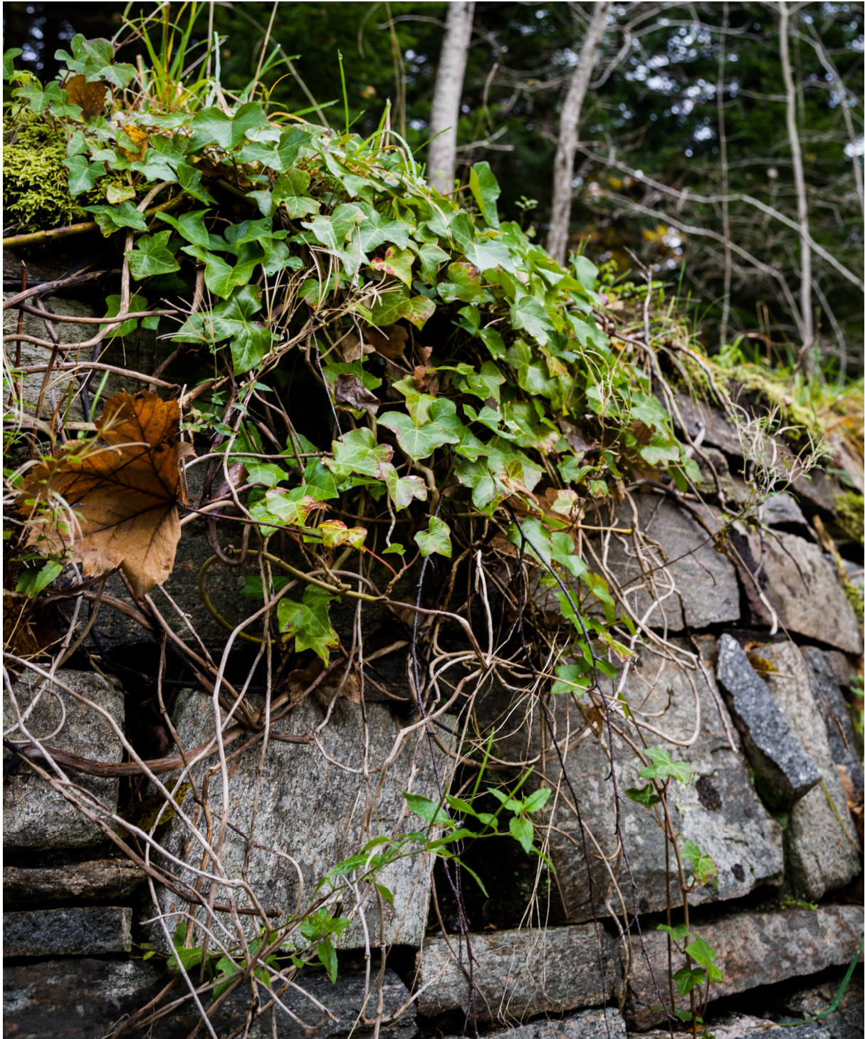
Figure 40 A stone wall that supports one of the terraces in Retiro. Apart from the raised paths and drainage channels, these stone walls are some of the more visible architectural structures. The wall has become a substrate for animals and plants. Despite the lack of upkeep and intrusive tree roots, the walls have impressively kept together well and are a testament to the understanding of the material by the mason that put them together. 16.10.2018, 11:48.
