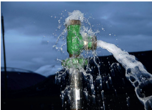
Figure 13. Artesian water from wellhead, producing 125 litres brackish water per minute from the Helvetiafjellet Formation, i.e., the upper aquifer.
