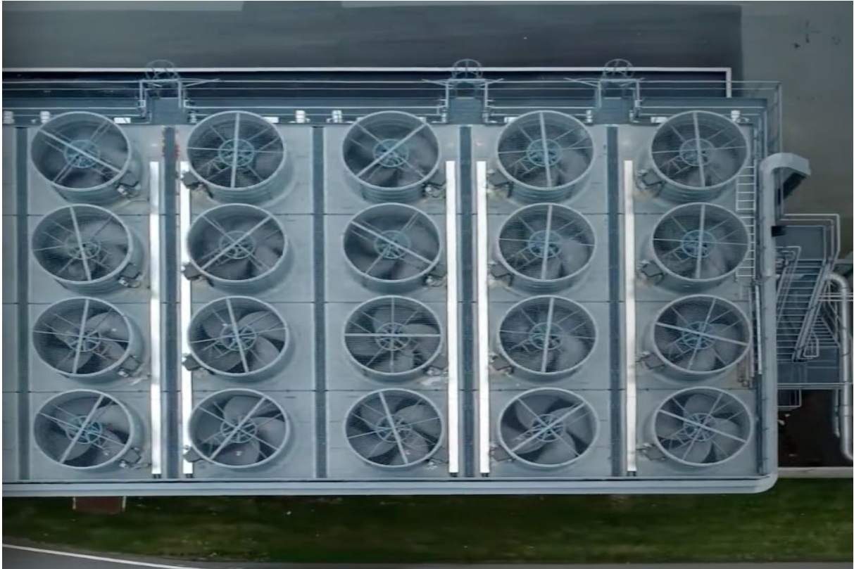
Figure 22. Aerial view of the condenser fans on the roof at Returkraft's plant [61].
