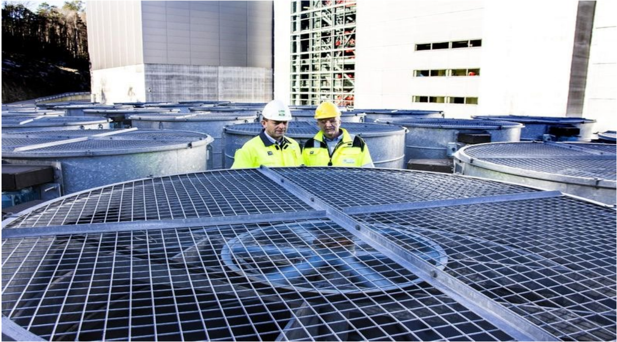
Figure 21. Condenser fans on the roof at Returkraft's plant used to discard excess thermal energy on the warmer months of the year. Photo: Tormod Flem Vegge [60].
