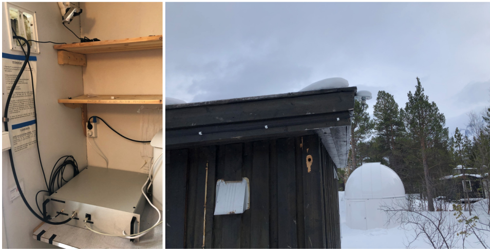
Figure 6.3: The rack mounted case as installed on the Skibotn site (left) and a partial photo of the hut it was installed in (right) where also the active GPS antenna can be seen mounted on the end of the roof.
