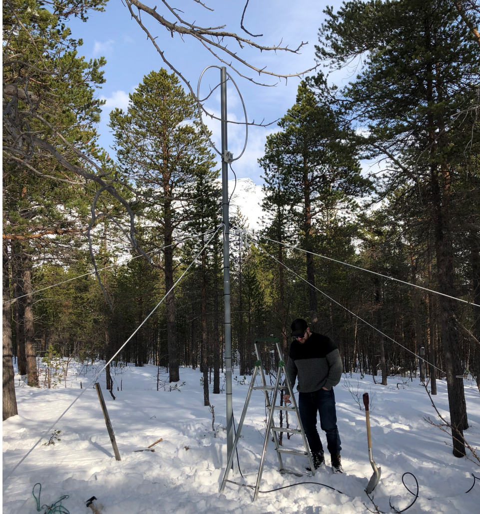
Figure 6.2: The Skibotn antenna installed using pine trees as fastening points for all four guy-wires.
