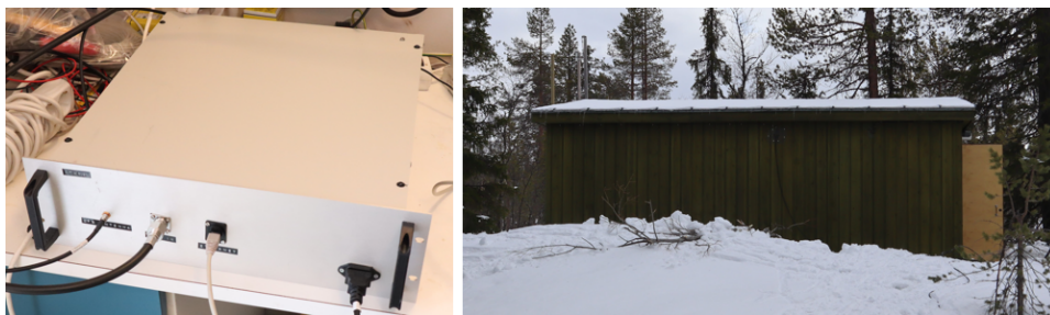
Figure 6.7: Photos from the Kuusamo site. Rack mounted case installed in the shack (left) and the instrument shack as seen from the outside (right). The GPS antenna can be seen mounted on piece of wood in the upper left corner of the shack image.
