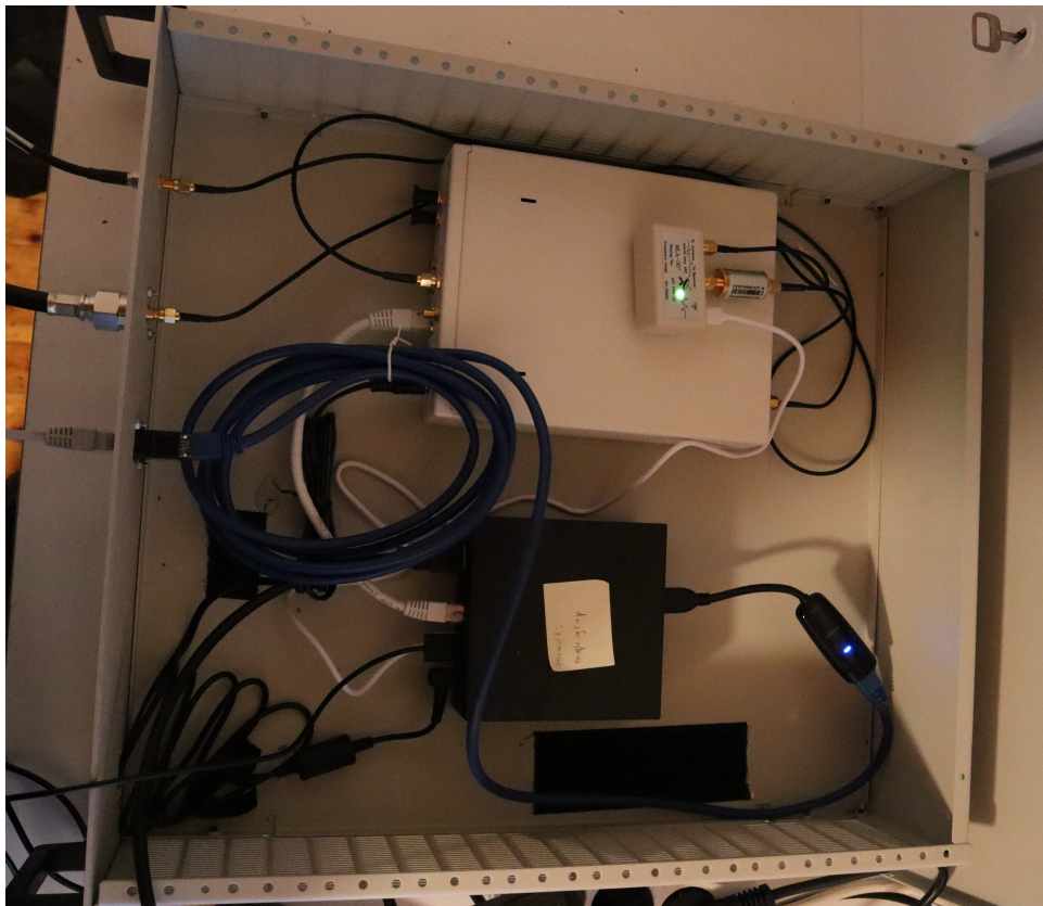
Figure 4.17: Overview of the rack mounted case with installed components.
