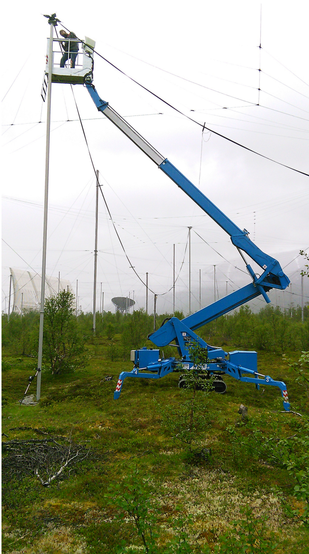
Figure 7. Repair work to one of the 12 m high antennas out of 144 such antennas in Array 1 to bypass existing and potential weak points in the twin-feed cable connection to the antenna centre. The original 23 m wooden masts are visible in the background. Note the different support mast and the different feed lines compared with the original design as used in Array 2 and Array 3, shown in Fig. 3. (Photo credit: Michael T. Rietveld)
