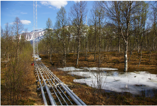
Figure 3. The fabricated coaxial cables and towers in one row of antennas of Array 2 in spring of 2010. The vertical tubes, which are part of the tower supporting the antenna, are also coaxial cables acting as quarter-wave transformers supplying the radio frequency (RF) current to the antenna. Array 3 has an identical design but is smaller in size. Originally, Array 1 had similar antennas, larger in size, but these were modified after the storm in 1985. (Photo credit: Michael T. Rietveld)
