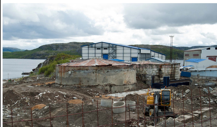
Fig. 11.3 Deteriorating storages for spent nuclear submarine fuel at Andreev Bay on the Kola Peninsula. Clean-up work is seen in front, and in the background are new buildings for the preparations for transit of this waste to a safer final deposit. Photo by Birgitte Wisur Olsen in 2015. Used by permission.
