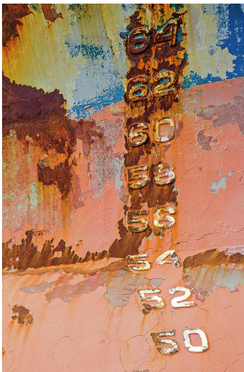
Figure 5: Faded paint and rusty draft scale [6]
