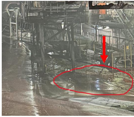
Figure 8: Ground water leakage on the tunnel floor-LKAB[11]
