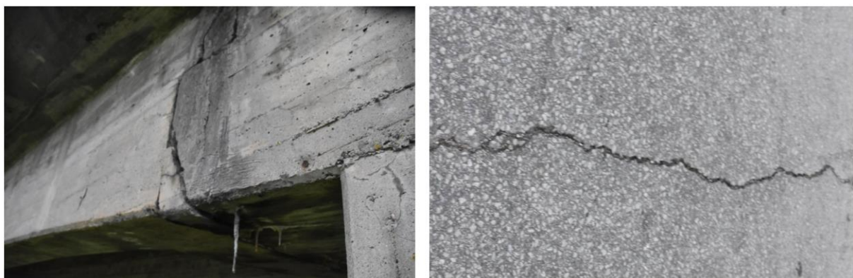
Figure 3-6: Photos of some of the cracks identified on Herøysund bridge
