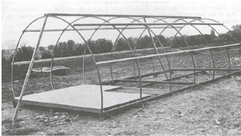
Fig.48 Stage 3. Wooden floor joists were screwed to the bearers to receive timber floor panels.
