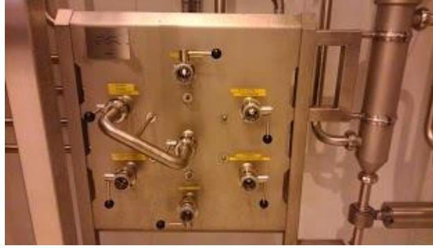
Figure 7: Flow plate at NAMAB that controls the product line through the facility.
