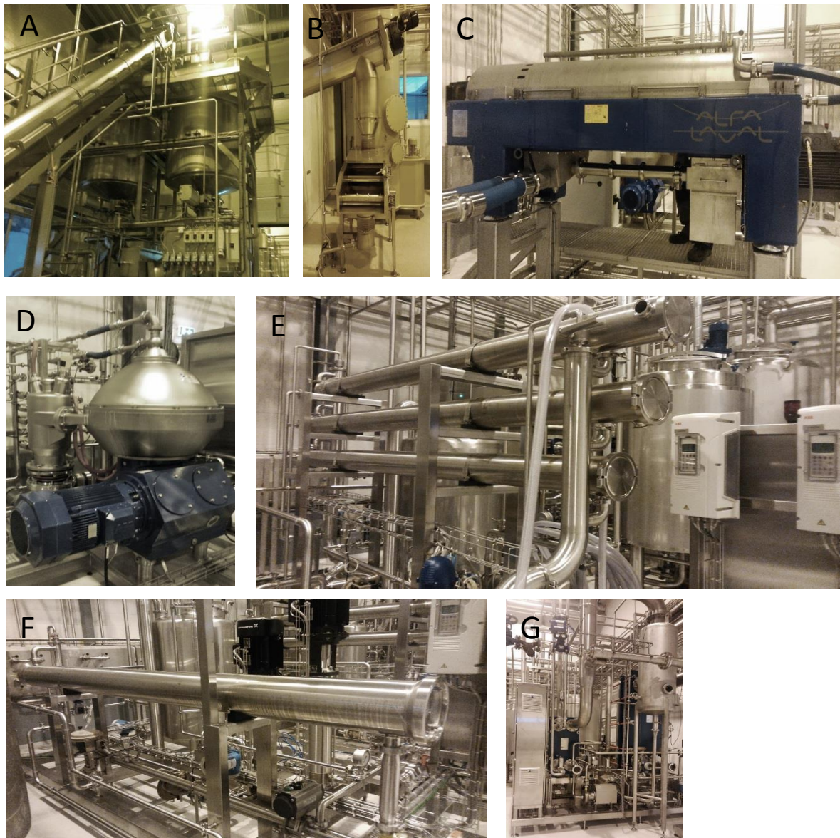
Figure 8: Components of the NAMAB facility. The raw material is fed into a grinder and then pushed up to the reaction tanks by a large conveyor screw (A), and then into the tanks by another conveyor screw which controls whether it goes into tank 1 or 2. From the reaction tank the hydrolysate, or possibly extract, is dropped into a container with a screw (not shown) where a coarse filtration of fluids and solids happen. The fluids are drained into a tank while the solids are pushed onto a shaking table (B) with a sieve that separates more fluids from the solids. The fluid continues to the decanter (C) where the material is separated into oil and stick water. In addition, smaller solid particulates are sorted out and dropped from the decanter into a mobile container. The oil, which floats on top of the stick water, is drained into one container and the stick water into another, similar container. The oil is pumped into an oil polisher/separator (not shown) where the last of proteins and other impurities are removed with the help of water. The stick water is pumped into a separator (D) where the last oil residues are removed. The oil can be transported back to the polisher. Both the clean oil and stick water is pumped into holding tanks. After going through the separator, the stick water can be ultra-filtered (E) and if need be, reverse osmosis filtered (F). The ultra-filtration system have three cylinders for the membrane filters (with a cut-off value of choice), which gives the possibility for relatively high throughput. The reverse osmosis system can remove molecules and ions from the solution by applying pressure to the system and forcing them through a semi-permeable membrane. Evaporators (G) can also be applied to concentrate the peptides in the stick water.
