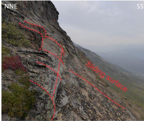
Figure 36: Potential sliding surface along fold limbs (red dashed line). Horizontal red dashed line represents fold axis. Location in bedrock region b1 (Fig.22).
