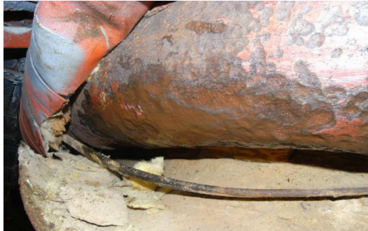
Figure 3.3: Picture showing an insulated and head trace pipe which have experienced CUI [Axess AS, 2015a].
