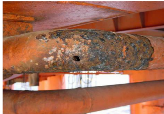
Figure 3.2: Internal corrosion on a well test pipe [Axess AS, 2015a].
