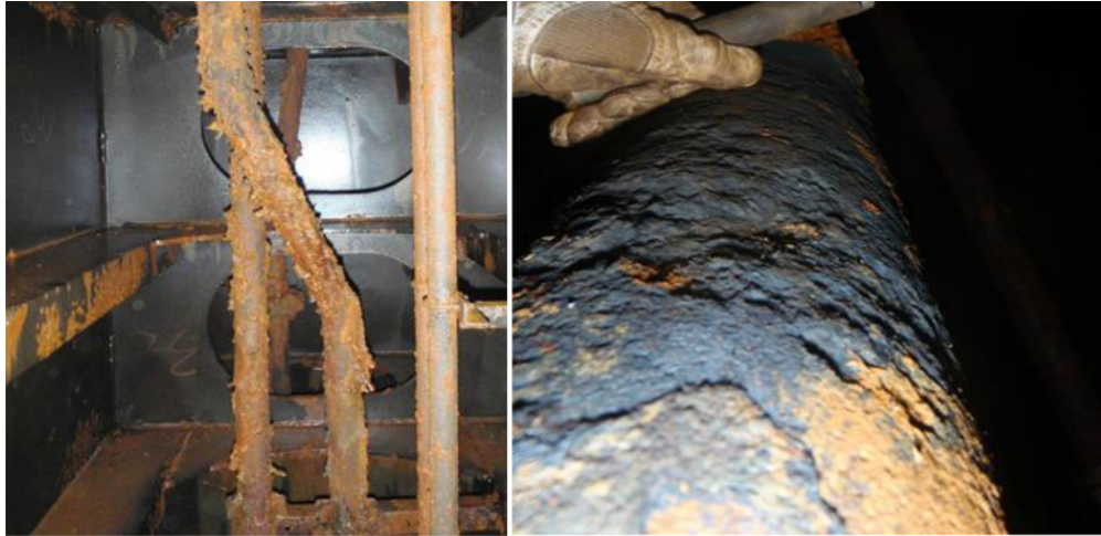
Figure 3.1: Picture showing general external corrosion on pipes through a ballast tank. Rust scale is removed on the picture to the right. [Axess AS, 2015a]
