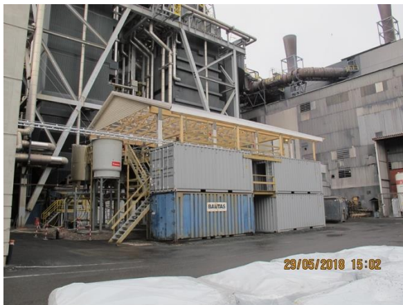
Figure 6: 300.000 litre tank inside Finnjord smelting plant (photo: Hans Christian Eilertsen)
