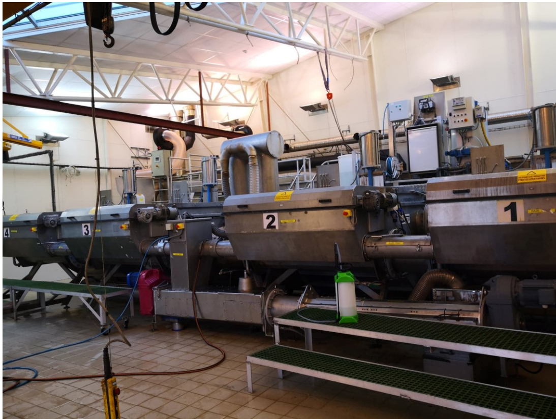
Figure 7. Breivika wastewater treatment station (private photo)
