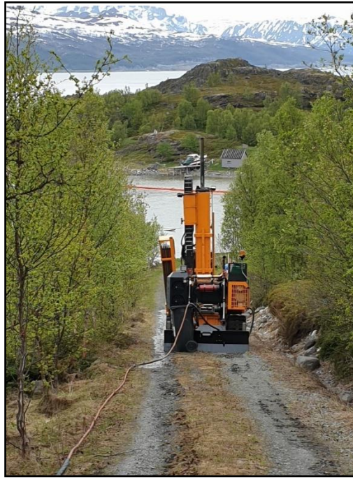
Figure 17: Photo of the hydraulic drill rig used at Kråknes. The rig is driven to the location by a remote operator. Photo: Multiconsult.
